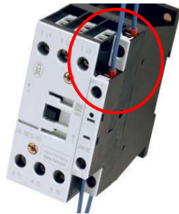
Control wiring terminals in the front
